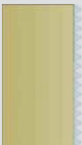
This leaves minute white/colourless crystals at the surface (known as Efflorescence)
